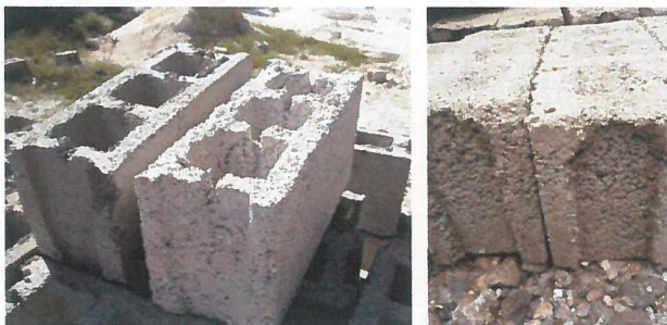
A rough finish at the top and sides of the block (right) is an indication of insufficient general compaction.
