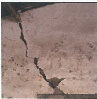
Concentrated roof load on poor masonry
